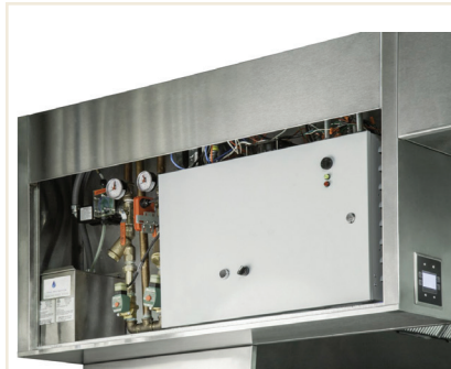
FIGURE 4 Valves, gages, and controls for electronic fire suppression and hood cleaning system in hood end cabinet.
