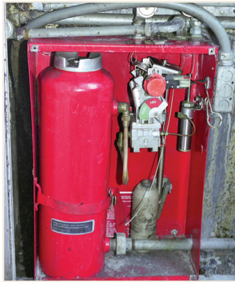
FIGURE 5 Fire marshal photo showing gas cylinder not installed in release mechanism.
